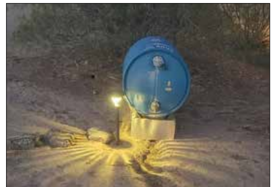
Pictured is Duvall North Water Station.
